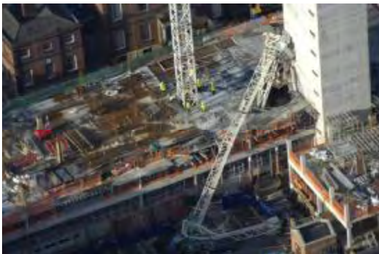
Liverpool crane collapse, 2007
