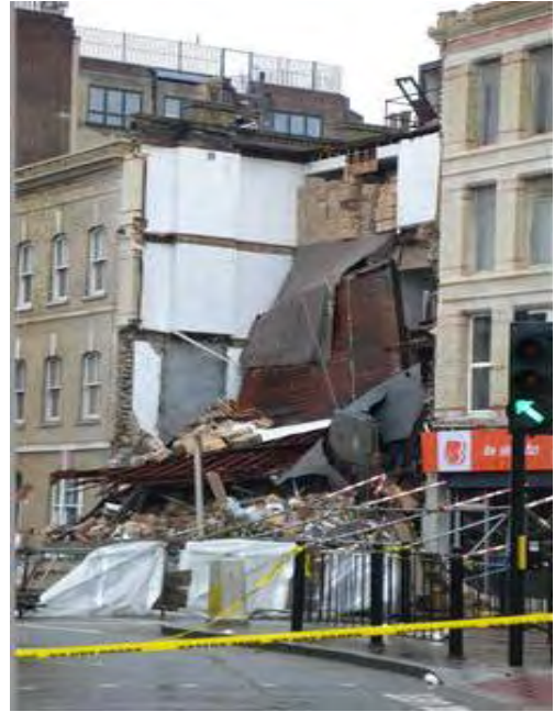
Commercial Rd collapse, London, 2007
