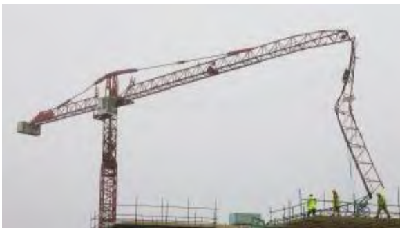
Durrington tower crane collapse, 2005
