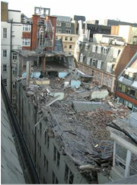
Dean Farrarh Street building collapse (aerial view) (courtesy HSE)
